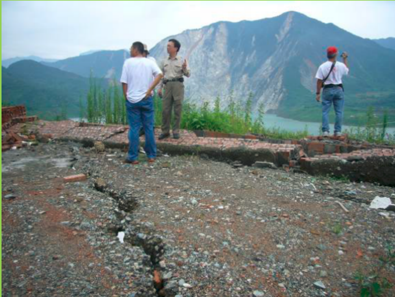
The right bank of the Minjiang River near Miaoziping of the Zipingpu Reservoir was cracked due to the earthquake 紫坪铺水库庙子坪附近岷江右岸受地震影响龜裂
