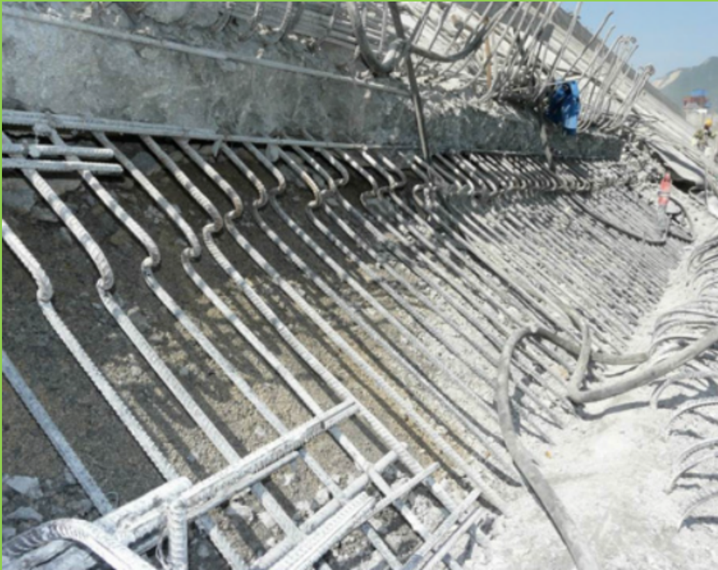
Dislocation damage observed after cleaning the damaged concrete 清洁损坏的混凝土后观察到位错损坏
