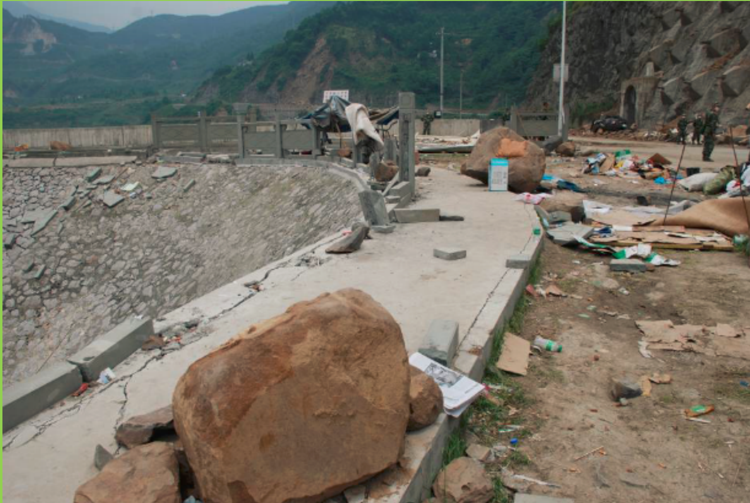
View of landslide boulders from the left slope of the abutment on the dam crown. 31^{\circ} 02' 08,89'' N – 103^{\circ} 34' 40,81'' E
